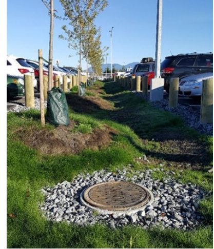
FIGURE 13: View of water filtering bioswale at YVR.
