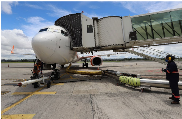
FIGURE 3: Brasília International Airport 400Hz in operation at airport's air bridges.
