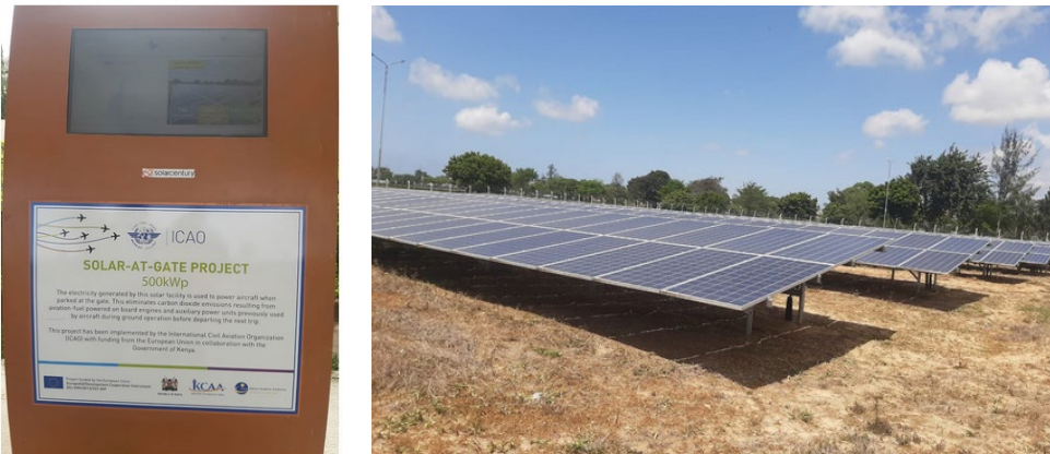
FIGURE 6: Solar Farm at Moi International Airport
