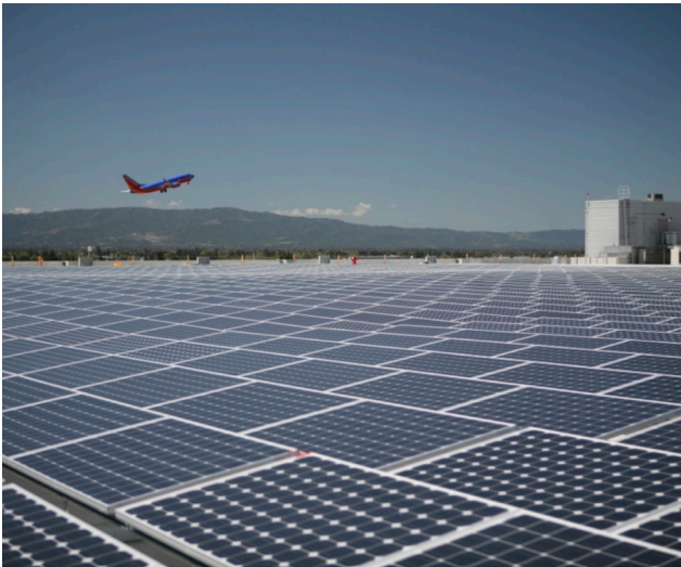
Figure 1. Solar at airport
