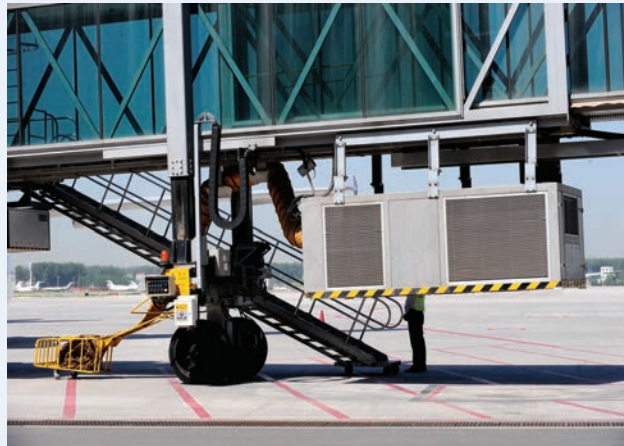
The CAAC endeavors to practice the specific program of "replacement of APUs usage by gate power units".
