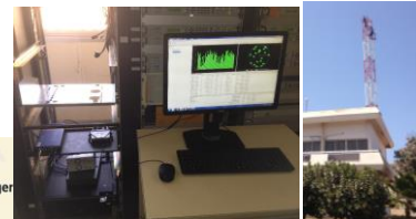
SAGAIE station (Dakar)
