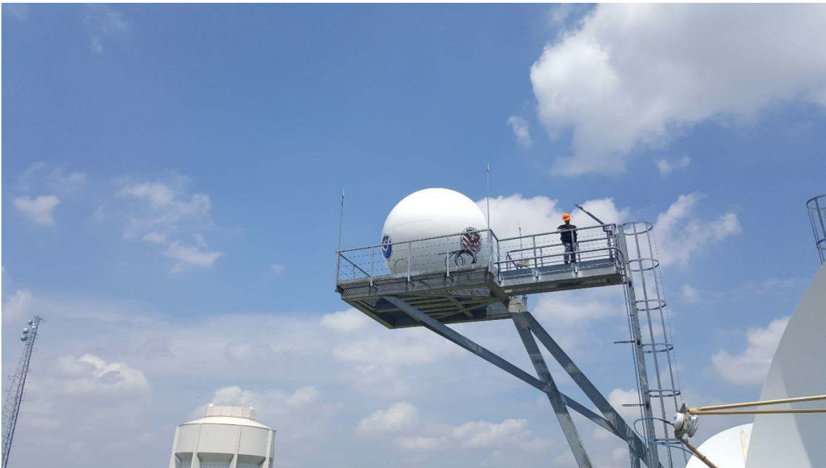
Figure 1: Installation of the antenna for Maryland Test LEOLUT (MEO channel)
