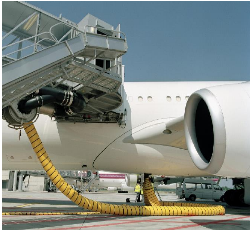
Ducting for Pre-Conditioned Air (PCA) – widely used many countries
