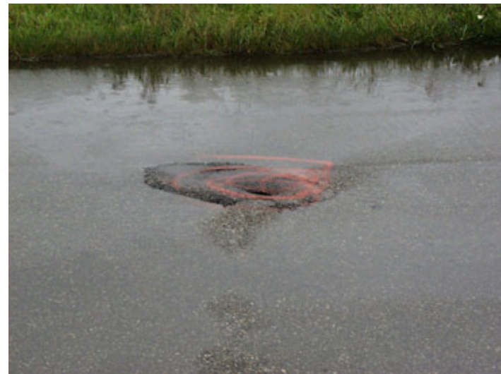
Flooding and subsidence beneath runway shoulder in Norway
