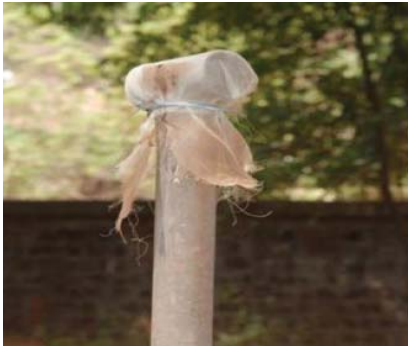
Figure 42. Distal end of vent pipe covered with nylon mesh prevents mosquito entry © Ashwani Kumar
