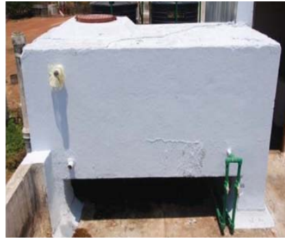
Figure 43. Vent pipe of an overhead tank covered with nylon mesh © Ashwani Kumar
