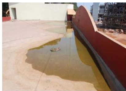
Figure 47. Blocked terrace with water © Ashwani Kumar
