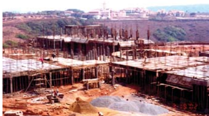
Figure 48. Construction site at PoE with an enormous potential for mosquito breeding © Ashwani Kumar
