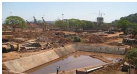
Figure 49. Water stagnation at new development site at a port © Ashwani Kumar
