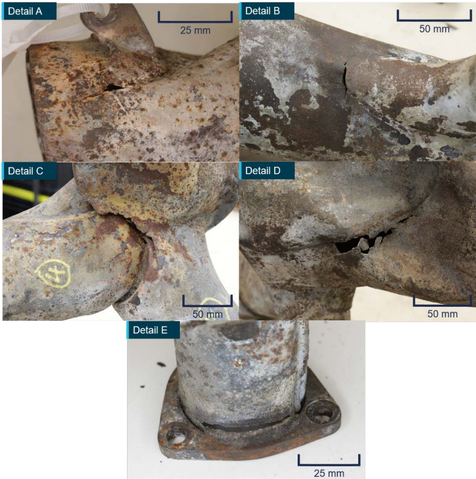
Figure 48: Detailed images of fractures identified in Figure 47 (scale approximate)
