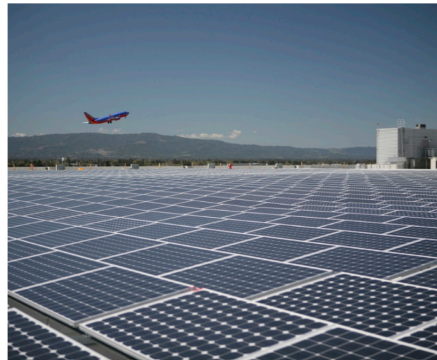
Figure 1. Solar at airport
