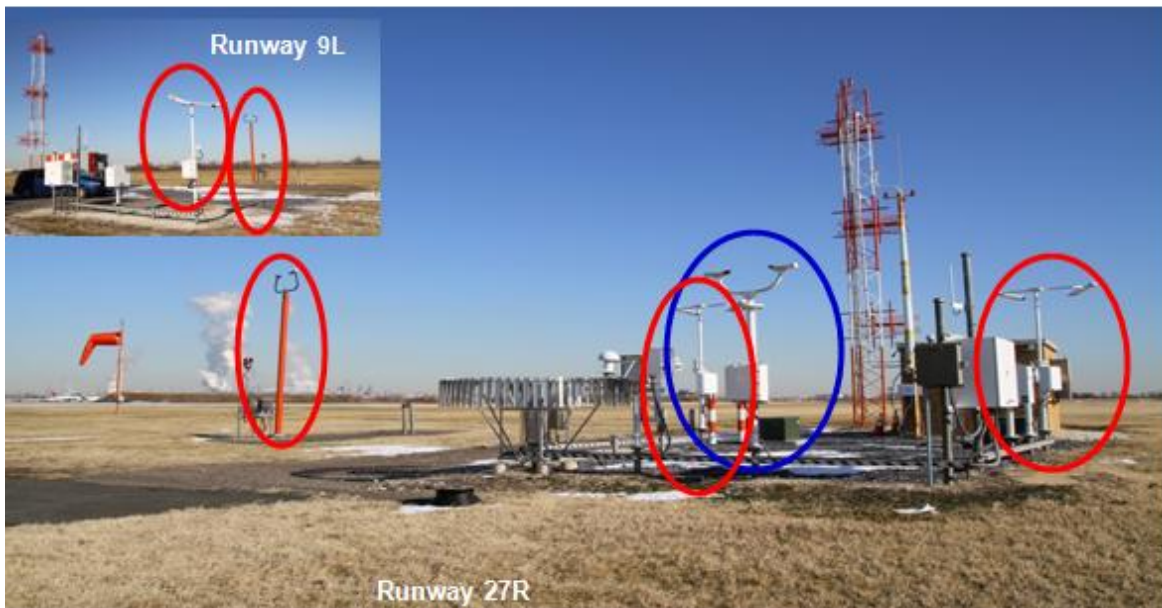
Figure 1. Close proximity of sensors at KPHL aerodrome. Red ovals are visibility sensors; blue oval is a present weather sensor. With today's technologies all can be consolidated while providing improved redundancy.
