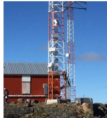
Figure 15: GBRT in Iqaluit w/ 4 Tx Antennas 7
