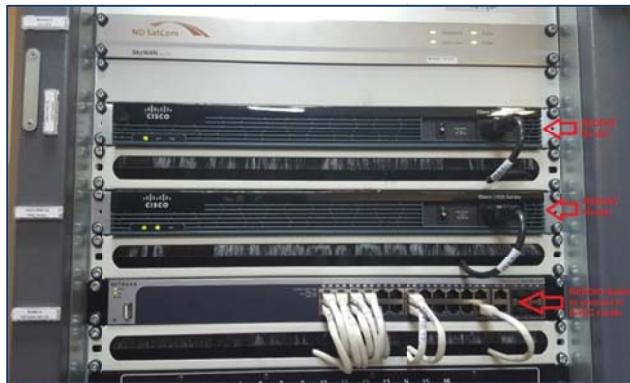
Figure 4: Node Santiago REDDIG Equipment.
