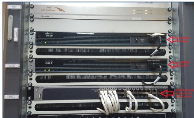
Figure 4: Node Santiago REDDIG Equipment.
