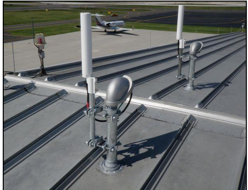
1090 and UAT Antennas
