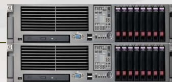
QUADRANTE Central Processor
