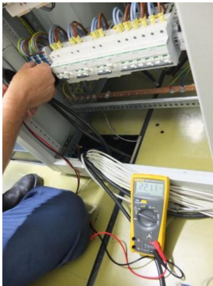
Figure 2 - Voltage measurement at the bay terminals
