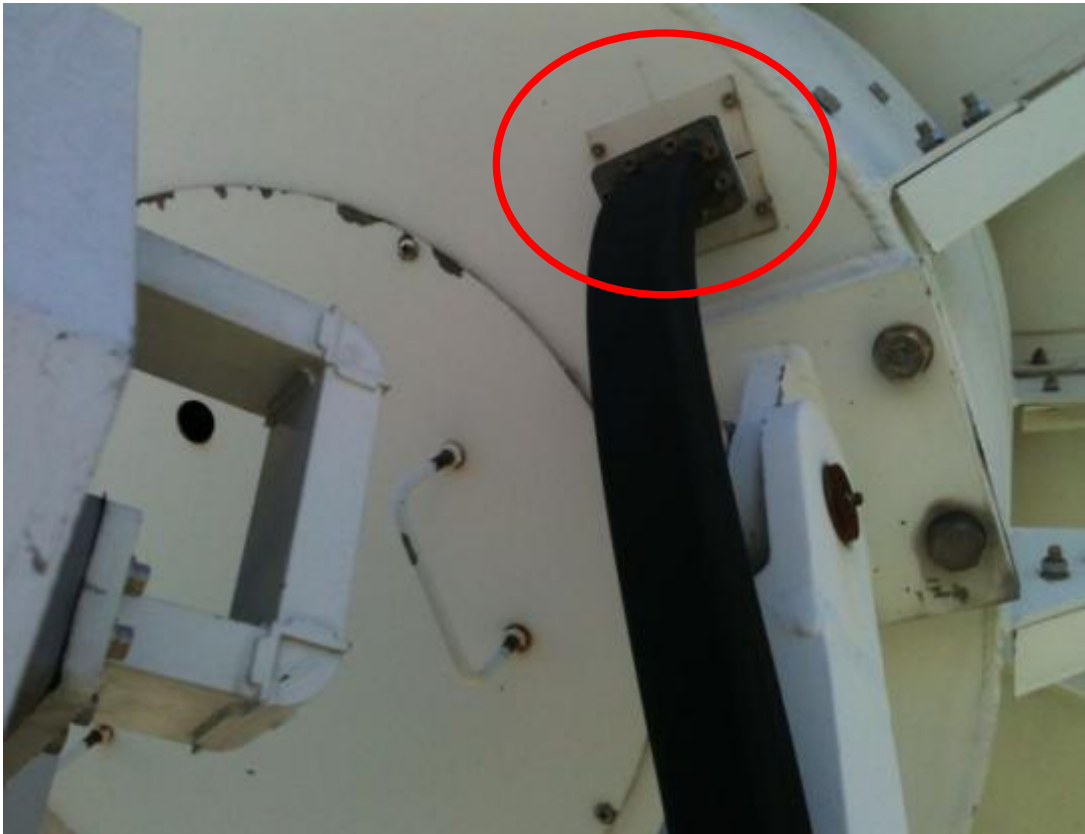
Figure 15 - View of the waveguide to be replaced
