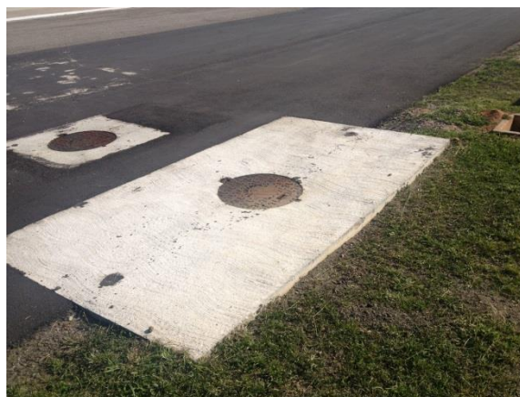
The manholes closer to the runway are now being corrected/ reinforced (heights/ cover types)
