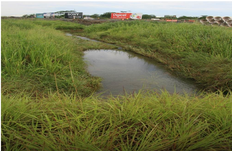
Drainage ditch overgrown with vegetation
