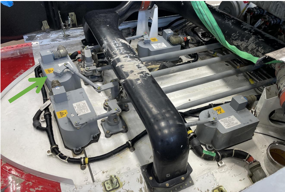
Figure 6: The four trim actuators installed on the upper deck above the cockpit on LN-OIJ. A green arrow points at the pitch trim actuator. Photo: NSIA
