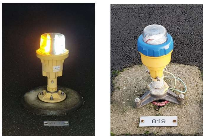
Figure 7: elevated runway edge lights (white/yellow) and elevated taxiway lights (blue)
