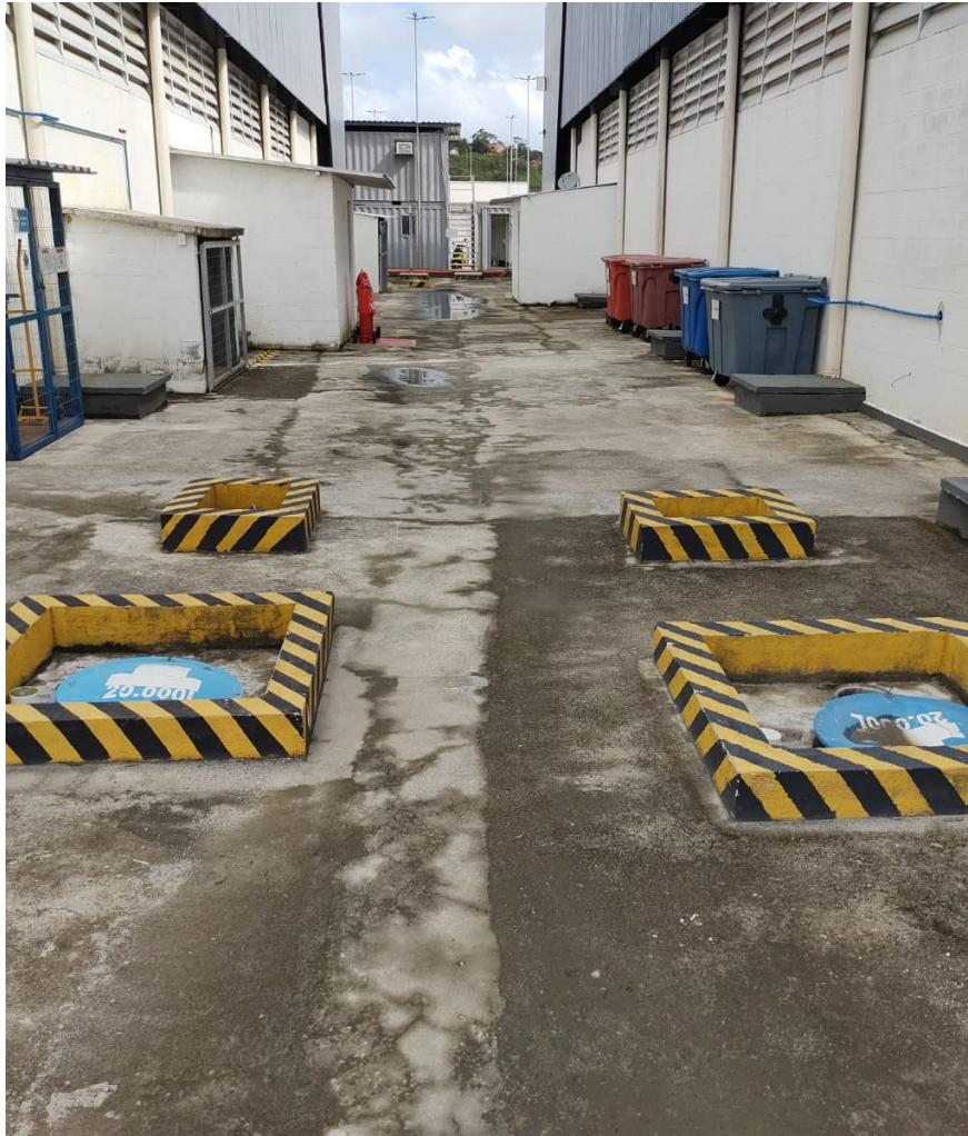
Rainwater harvesting – Maricá Airport
