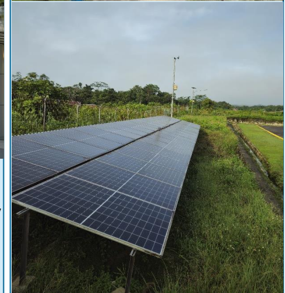
Solar PV at Ayawasi Airport, Cap. 120 KVA Operated on Dec 2021
