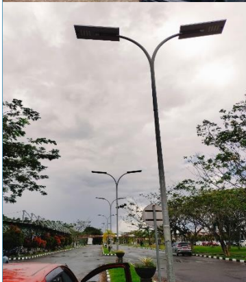
Solar powered lights, Access road Cap. 50 @60watt Operated on May 2021
