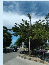
Solar powered lights, At air side and access road Cap. 75 @60watt Operated on Dec 2022
