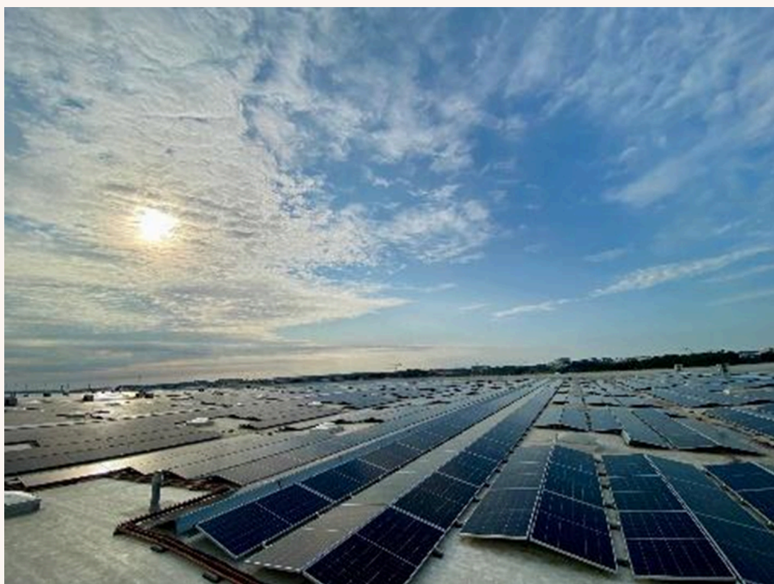
Figure 7. Brussels Airport Cargo: A new installation of 65.000m 2 of solar panels (7.3 MW) covering the roof of our newest building at Brucargo.
