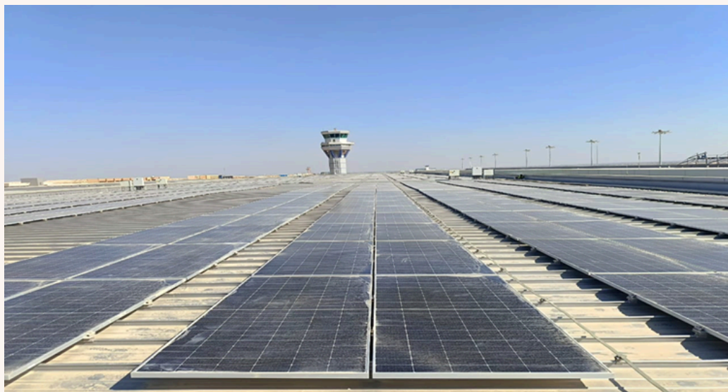
Figure 9. Borg El Arab International Airport – Solar farm on the terminal phase 2 with capacity 1.4 Mw
