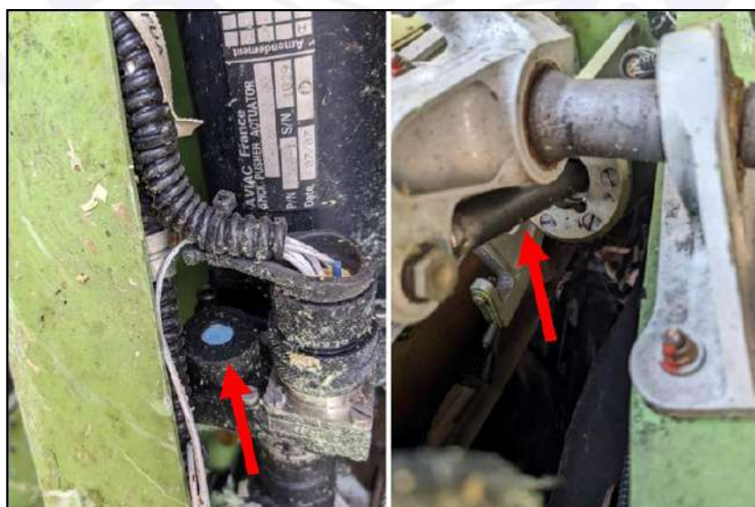
Figure 90 – On the left, a red arrow indicating the desiccant cartridge in blue; on the right, a red arrow indicating the extended position of the actuator rod, consistent with the non-actuated condition.
