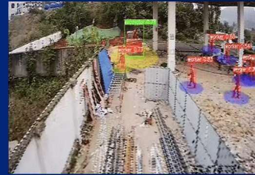
Construction Safety Hazard Identification
