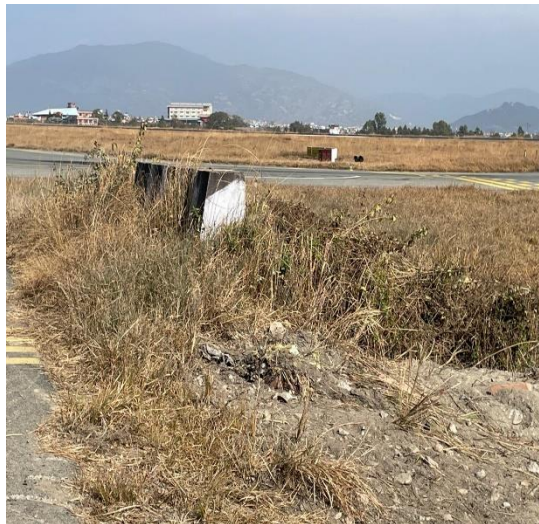
Figure 2: Elevated side wall near taxiway strip
