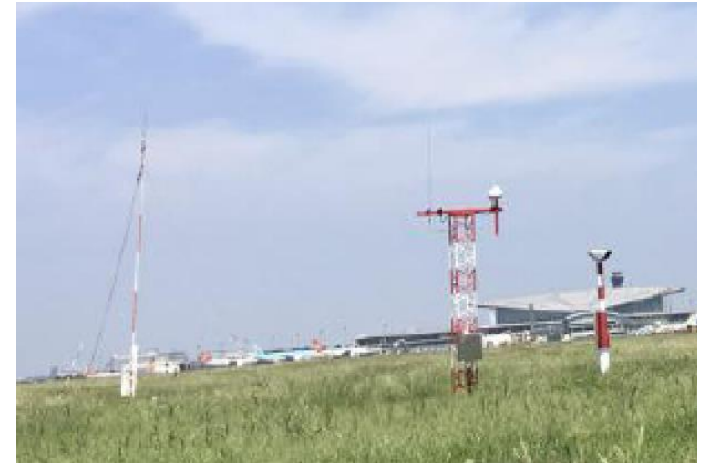
GBAS stations in China (Tianjin and Lhasa)
