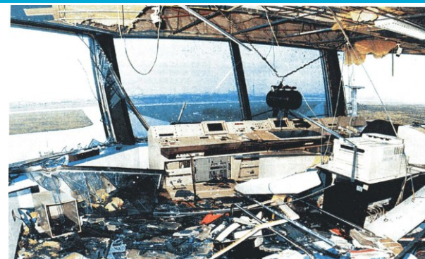
Damaged Control Tower
