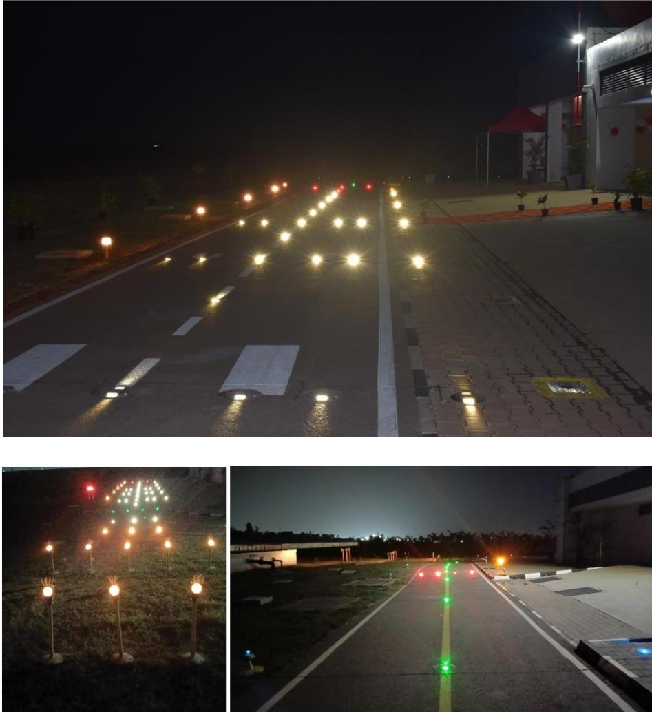
Fig 1. Demo Runway with lightings provided at KIA- AGL training centre
