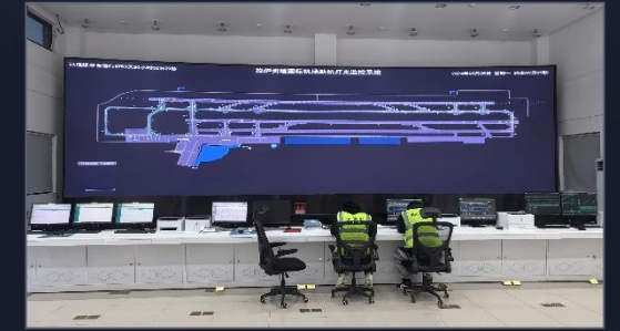
Smart lighting system
