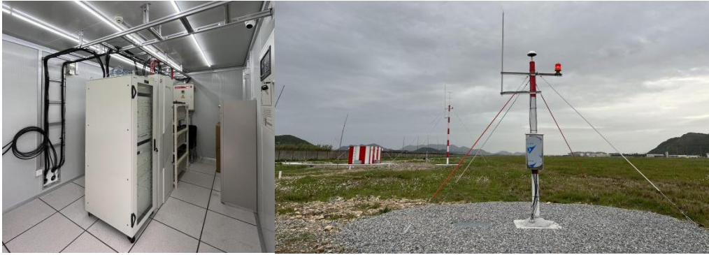
Figure 1. Outdoor equipment of GBAS ground station
