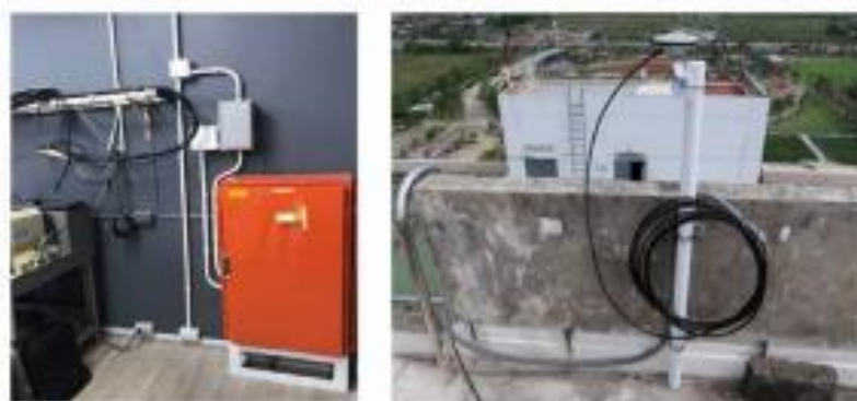
Figure 4. IFM Antenna and Receiver installed at KMITL
