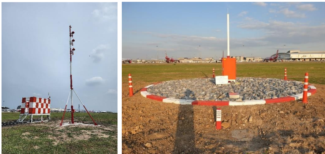
Figure 3. GBAS Shelter and VDB antenna (left) and RR antenna (right) installed at Suvarnabhumi International Airport
