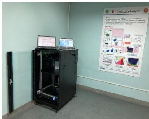
GNSS Data Analyzer in Philippine CATC equipment room
