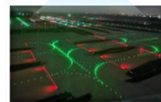
Taxiway center line lights Stop bars
