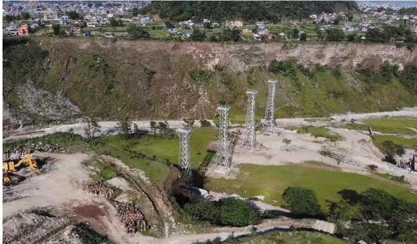
Figure: 4 Tower for installation of Approach lighting system as seen from the bank of the river
