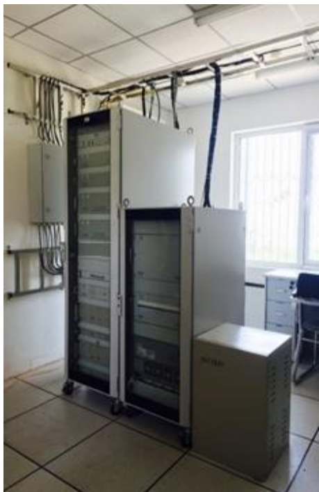
Main Station equipment cabinet
