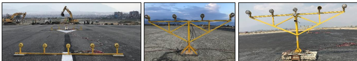
A) VNKT B) 1909110615 C) 1912102359 E) EXISTING APPROACH LIGHT CROSS BAR LIGHTS AT 300 M FROM THR 02 IS RELOCATED AT 310 M FROM THR 02 PILOTS TO ECT/ECL
