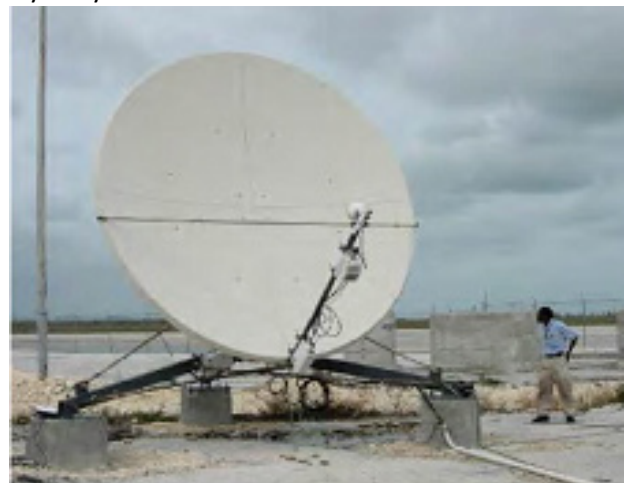
Flyaway antenna 3.8 meters
