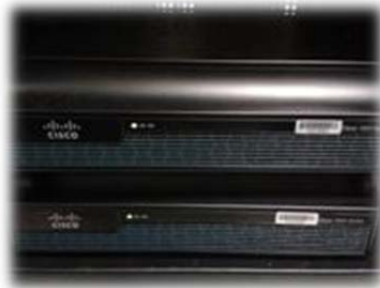
Routers installed by the service provider
