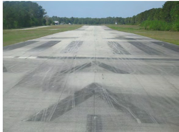
FIGURE 4-13. MARKINGS ARE OBSCURED BY ALGAE.
