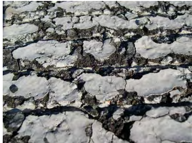
FIGURE 4-5. MAGNIFIED PHOTO OF FIGURE 4-4 SHOWS CRACKED ASPHALT WHERE WATER INVADES.
