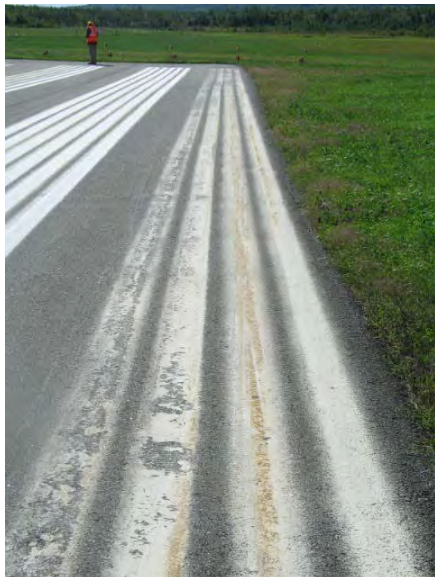
FIGURE 6-16. LAYERED STRIATIONS ON THE SIDELINE WERE SCRAPED OFF BY SNOWPLOWS.
