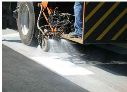
FIGURE 6-47. GLASS BEAD DISPENSERS ADJUSTED TOO HIGH.
