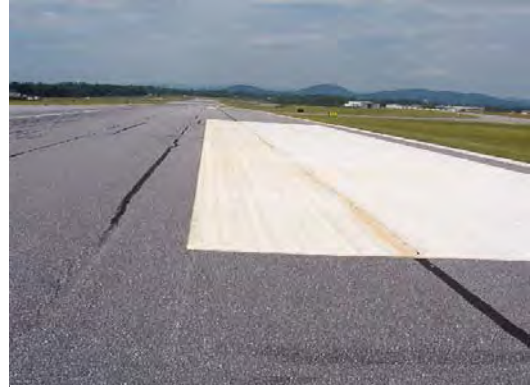
FIGURE 6-13. JOINT MATERIAL DISCOLORS THE WHITE PAINT.
