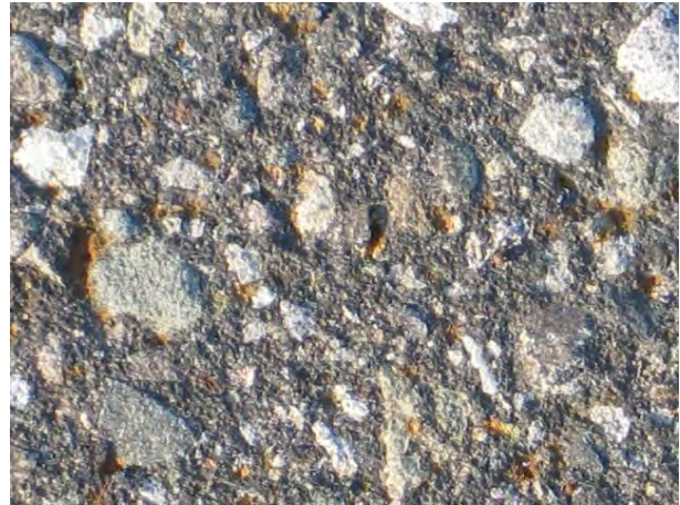
FIGURE 5-15. A CLOSE-UP OF FIGURE 5-14 SHOWS RUST AREAS WHERE SHOT REMAINED.
