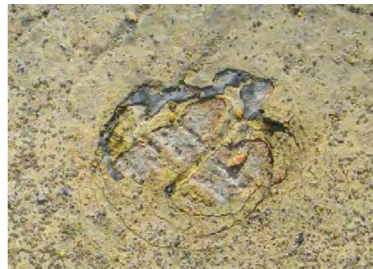
FIGURE 6-7. MULTIPLE LAYERS OF PAINT FILL THE GROOVES.
