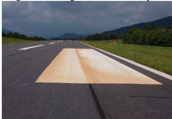
FIGURE 4-24. STAINED LEADING EDGE AND LOW AREA ALONG JOINT WHERE WATER FLOWS.
