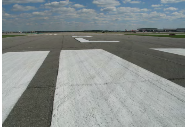
FIGURE 6-38. THE SAME MARKING AS IN FIGURE 6-37 DURING DAYLIGHT.
