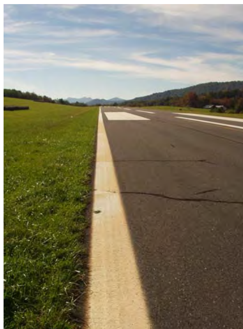
FIGURE 4-43. RUST STAIN BLED THROUGH NEW COATING.
