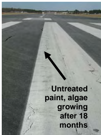
FIGURE 4-18. PAINT USED WAS STANDARD TT-P-1952E.
