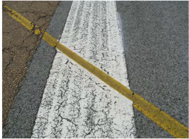
FIGURE 5-3. CRACKED AND PEELING MARKINGS – REMOVE 85 PERCENT.
