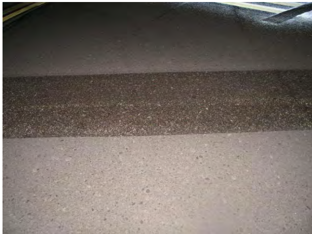
FIGURE 5-20. A SCAR FROM ULTRA-HIGH-PRESSURE WATERBLASTING ON GOOD ASPHALT.
