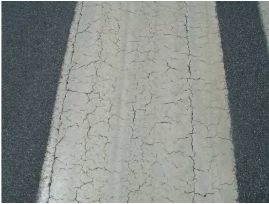
FIGURE 4-6. THIS MARKING IS 30 MONTHS OLD AND CRACKED.
