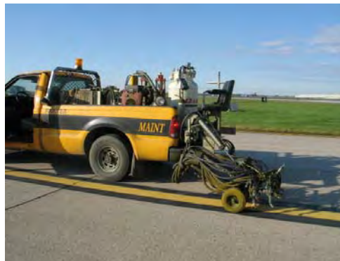
FIGURE 6-22. SKID MOUNTED PAINT RIG APPLIED BLACK BACKGROUND FOR TAXIWAY CENTERLINE IN FIGURE 6-23.
