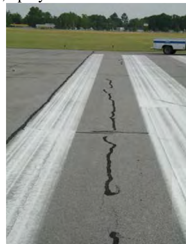
FIGURE 4-15. THE SAME SIDELINE AND THRESHOLD MARKING EIGHTEEN MONTHS LATER.
