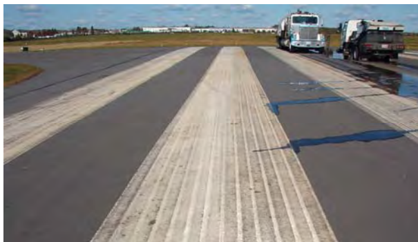
FIGURE 4-1. BEFORE CLEANING LOOSE AND POORLY BONDED PAINT.
