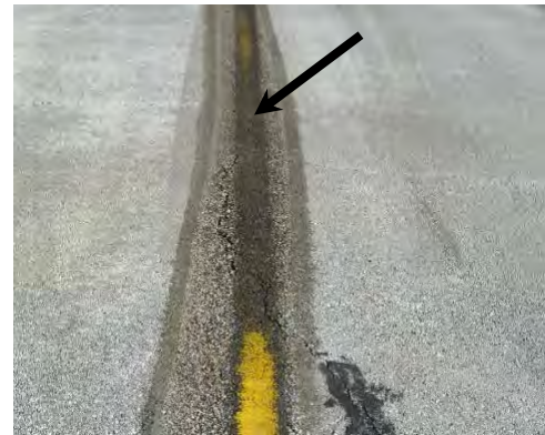
FIGURE 5-26. THE SCAR IS THE DARK PORTION OF THE ASPHALT THAT WAS SHIELDED FROM UV.
