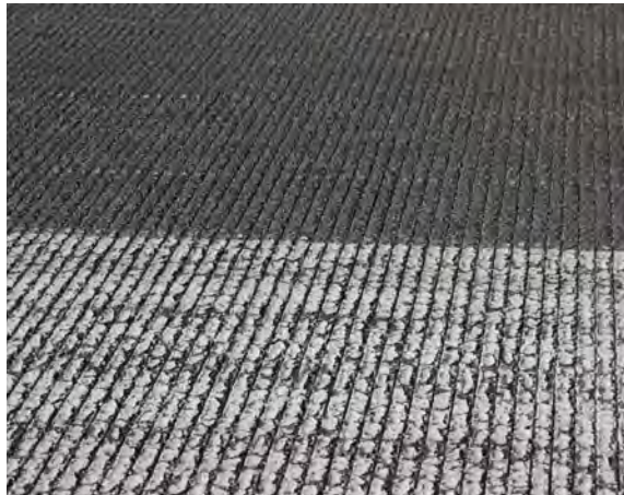
FIGURE 4-4. REPEATED PAINTING ON ASPHALT RESULTS IN PAINT BUILD UP, AND CRACKING OF PAINT AND PAVEMENT.
