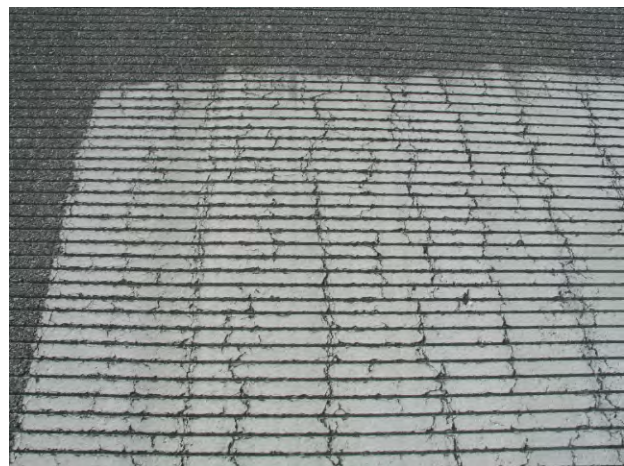
FIGURE 6-12. THE HEAVIER PAINT IN THE OVERLAP AREA CAUSED THE PAINT AND THE ASPHALT TO CRACK.
