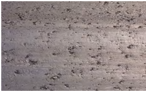
FIGURE 4-9. BEFORE RUBBER REMOVAL.
