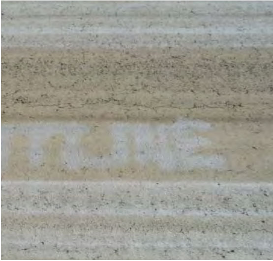
FIGURE 4-30. RUST REMOVER WHITENS STAINED MARKING WHERE “TLINE” WAS PRINTED.
