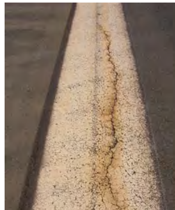
FIGURE 4-27. EVIDENCE OF RUST CONTAMINATION FROM SUBSTRATE.
