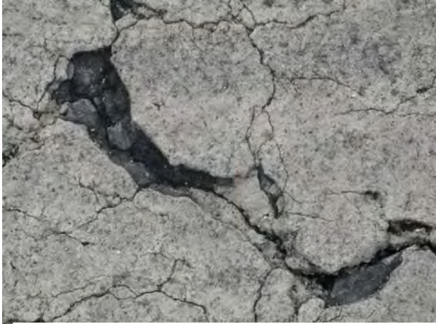
FIGURE 5-29. CRACKED PAINT INDICATES PRE-EXISTING PAVEMENT DETERIORATION.
