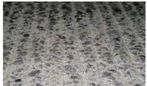
FIGURE 5-17. AFTER TEN YEARS OF SHOTBLASTING TO REMOVE RUBBER DEPOSITS.
