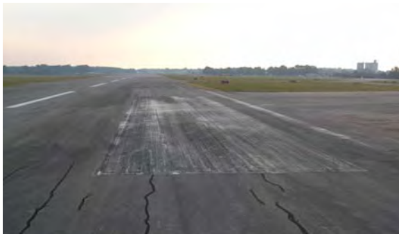
FIGURE 4-16. BEFORE WATERBLASTING: ALGAE OBSCURE MARKING.
