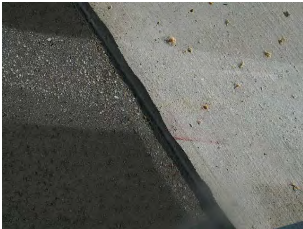
FIGURE 5-14. USED FOR REMOVAL ON NON-GROOVED SURFACES, SHOTBLASTING CAN BE A BEST PRACTICE.
