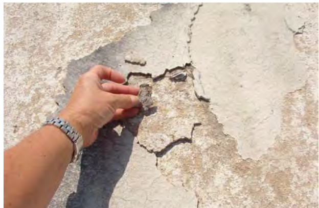
FIGURE 5-6. HEAVY PAINT BUILD UP ON CONCRETE.
