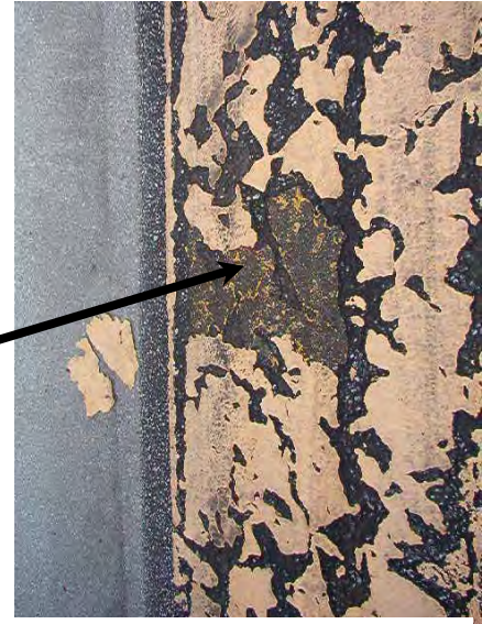
FIGURE 6-11. ENLARGED PORTION OF CRACKED ASPHALT.
