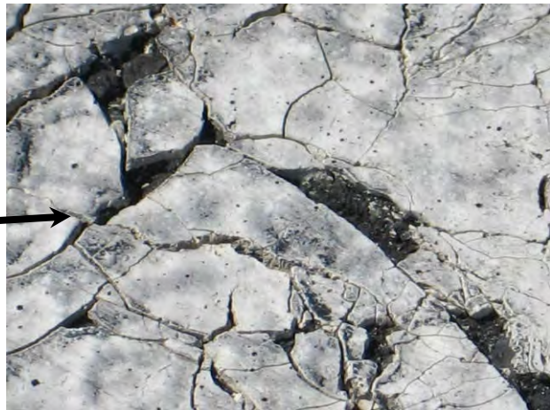
FIGURE 6-9. THICK COATING CRACKED, CAUSING PAVEMENT TO CRACK AS WELL.
