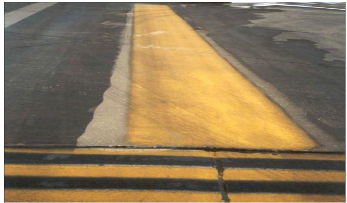
FIGURE 4-36. TAXIWAY SHOULDER MARKING WAS CONTAMINATED WITH OILY JET BLAST.
