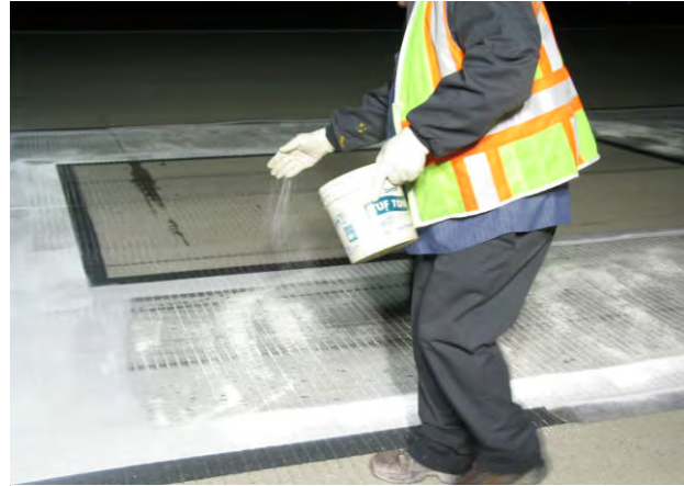
FIGURE 6-33. HAND-THROWN GLASS BEAD APPLICATION IS UNEVEN, POORLY DISTRIBUTED, AND POORLY EMBEDDED.
