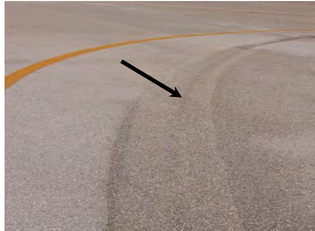
FIGURE 5-19. REMOVAL DONE ONE YEAR EARLIER; THE DARK SCAR HAS OXIDIZED AND FADED.
