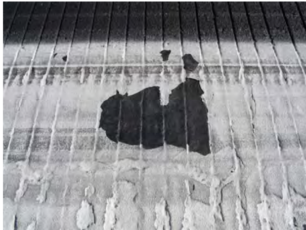
FIGURE 5-7. PAINT IS PEELING OFF OF REJUVENATOR APPLIED OVER OLD MARKINGS.
