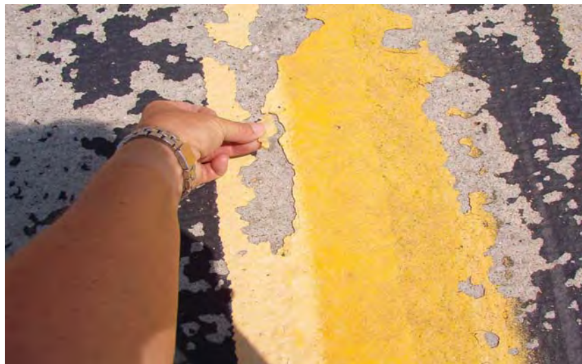
FIGURE 4-42. LOOSE PAINT FOUND AFTER SURFACE PREPARATION. PAINT REMOVAL IS REQUIRED.
