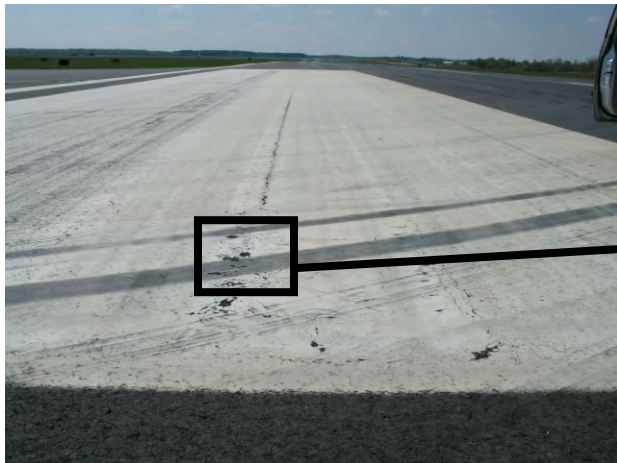
FIGURE 6-8. TOO MUCH PAINT WAS APPLIED IN OUTLINED AREA.
