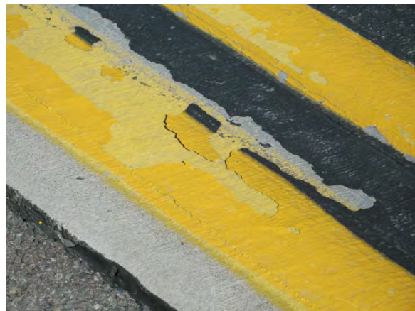
FIGURE 2-1. PEELING PAINT LAYERS
