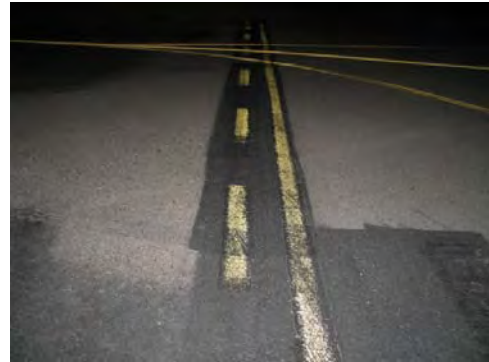
FIGURE 5-1. BLACKED-OUT NON-MOVEMENT BOUNDARY LINE IS VISIBLE AT NIGHT.
