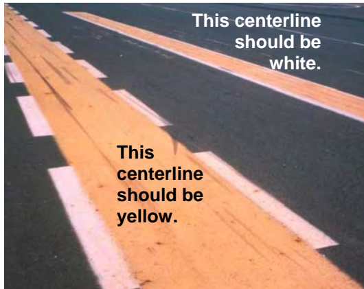
FIGURE 4-26. WHITE CENTERLINE LOOKS YELLOW.
