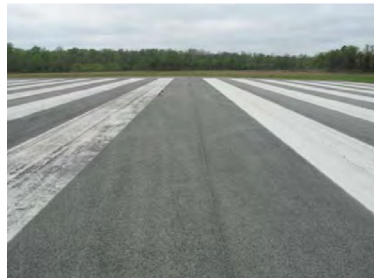
FIGURE 4-20. SAME MARKINGS AS IN FIGURES 4-18 AND 4-19, AFTER THIRTY MONTHS.
