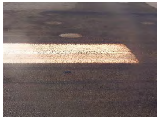
FIGURE 4-33. ANOTHER VIEW OF THE OIL-STAINED MARKING IN FIGURE 4-32.
