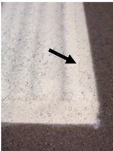
FIGURE 4-11. PAINT CRACKS WHEN APPLIED TOO THICKLY.
