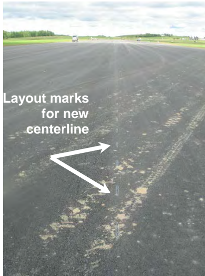
FIGURE 6-2. CONSTRUCTION DIRT MUST BE CLEANED.
