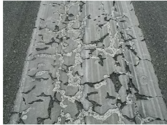
FIGURE 4-7. MANY LAYERS OF PAINT ON ASPHALT.
