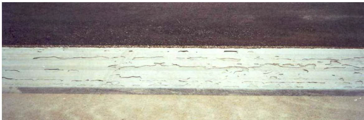
FIGURE 4-3. REPEATED PAINTING ON CONCRETE LEADS TO FOD.
