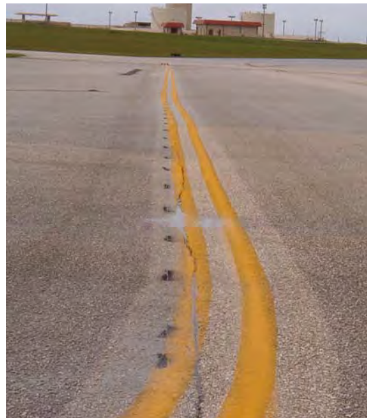
FIGURE 2-4. MARKING IS OUT OF ALIGNMENT
