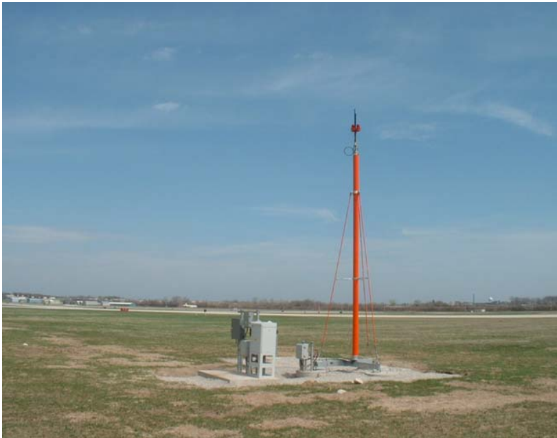
Figure 7 -- Sample Mode S Multilateration and 1090ES ADS-B Ground Station Installation for FAA ASDE-X Program.
