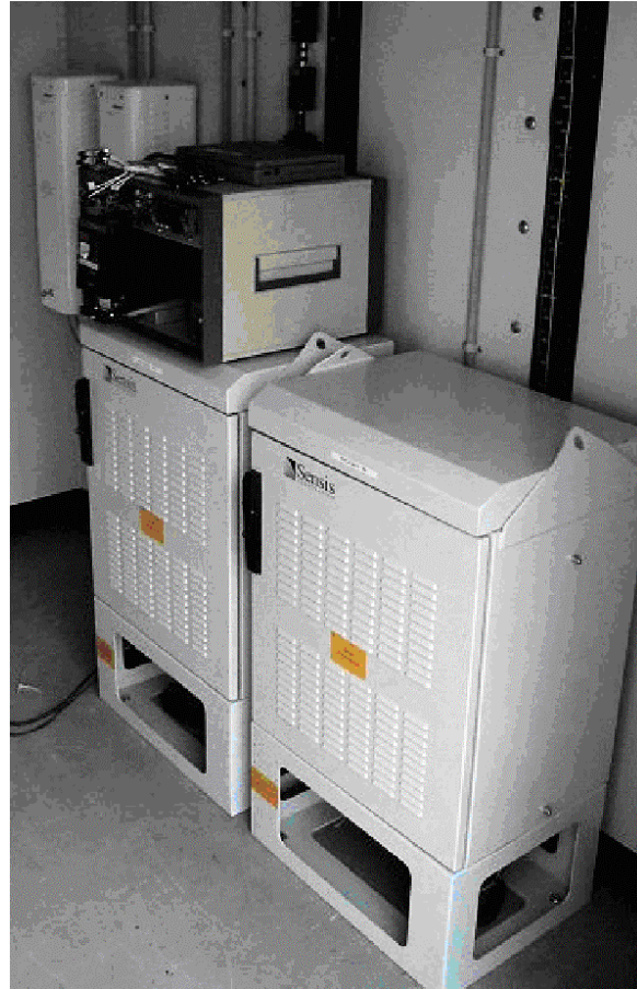
Figure 2 -- Redundant Mode S 1090ES ADS-B Ground Stations Installed In An Shelter At Base of Communication Tower NASA HITS/GOMEX ADS-B Trial
