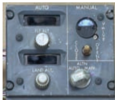
The digital pressure control panel of the B737-300. The AUTO and ALTN positions provide automatic cabin pressure control, while the MAN position allows manual control
